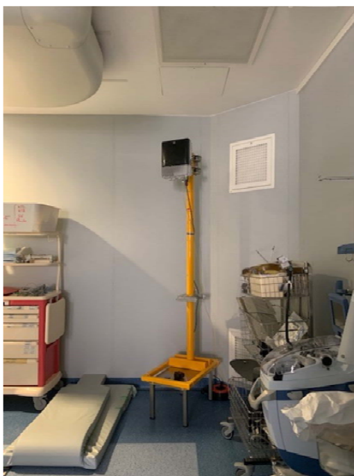
Figure 105. 5G antenna placement in the surgery room.
