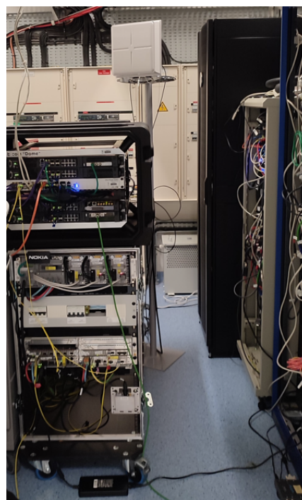
Figure 89. TheraImage technical room.
